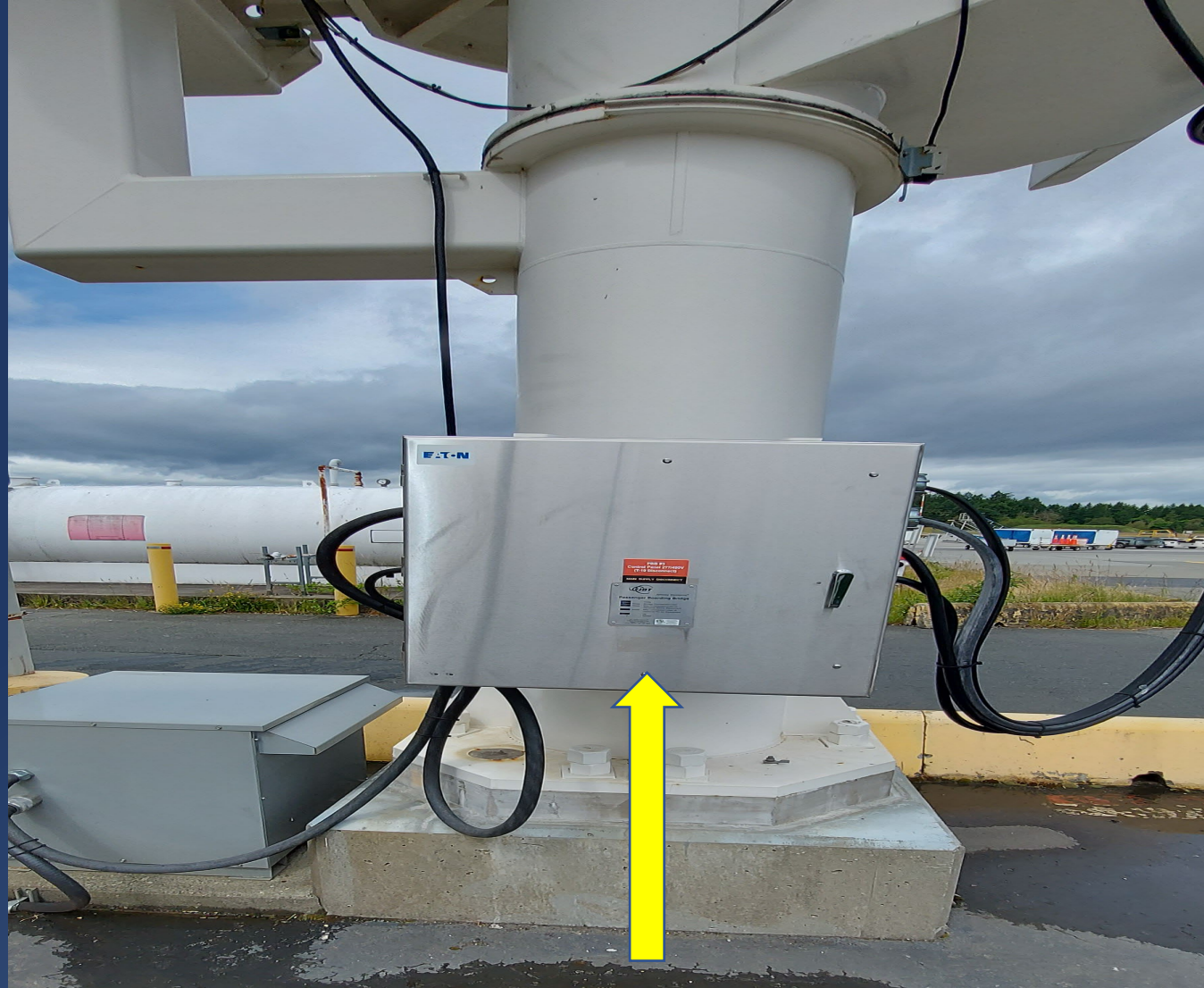
Main Power Disconnect Panel
