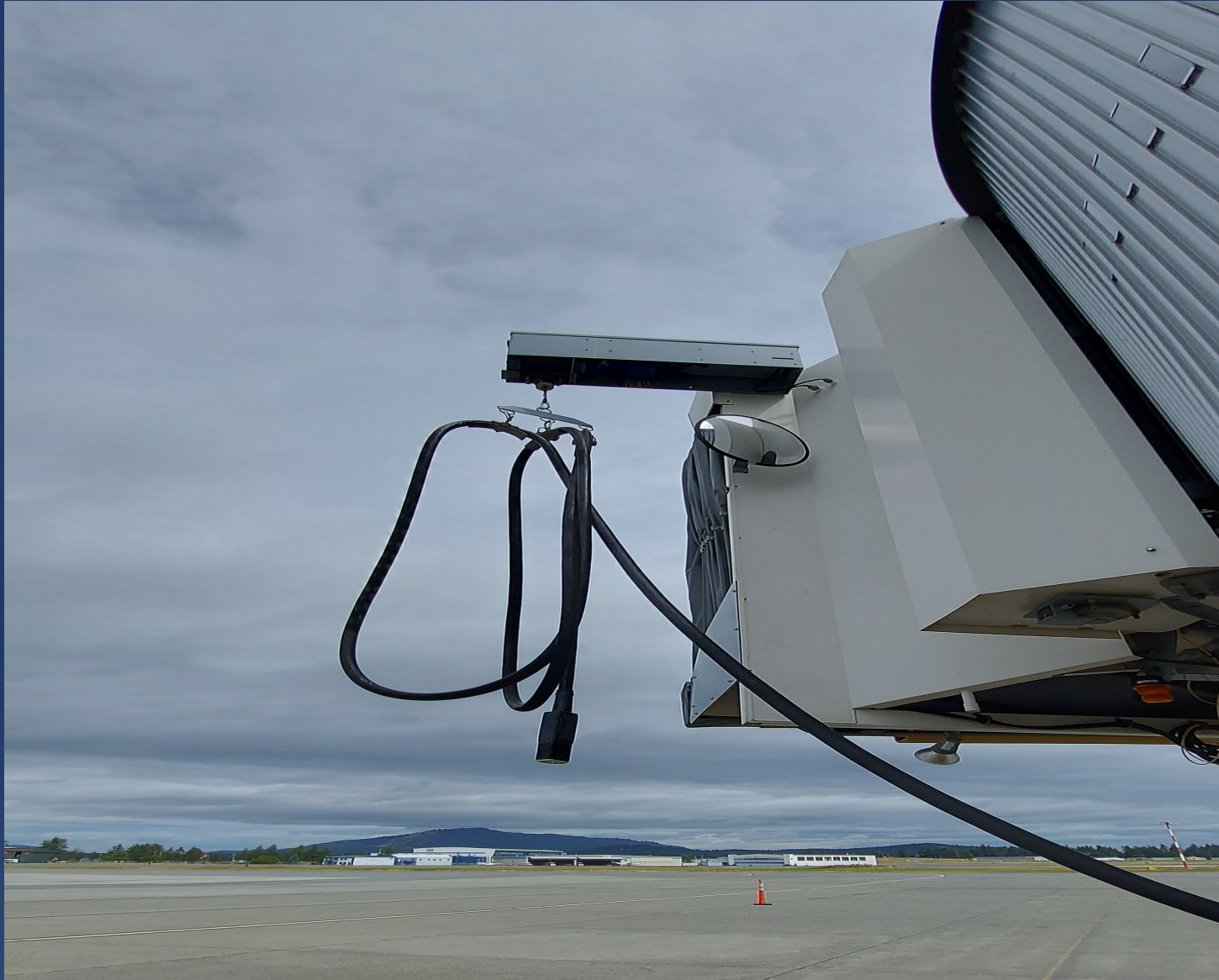
The ground power cable
